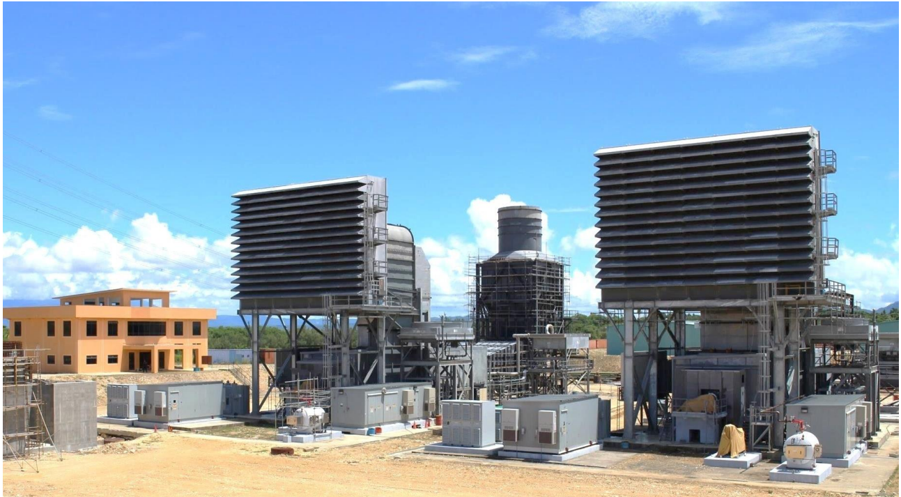
Philippines Power Plant 2 x 200MW
