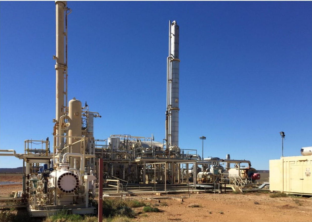
Eromanga Gas Plant
