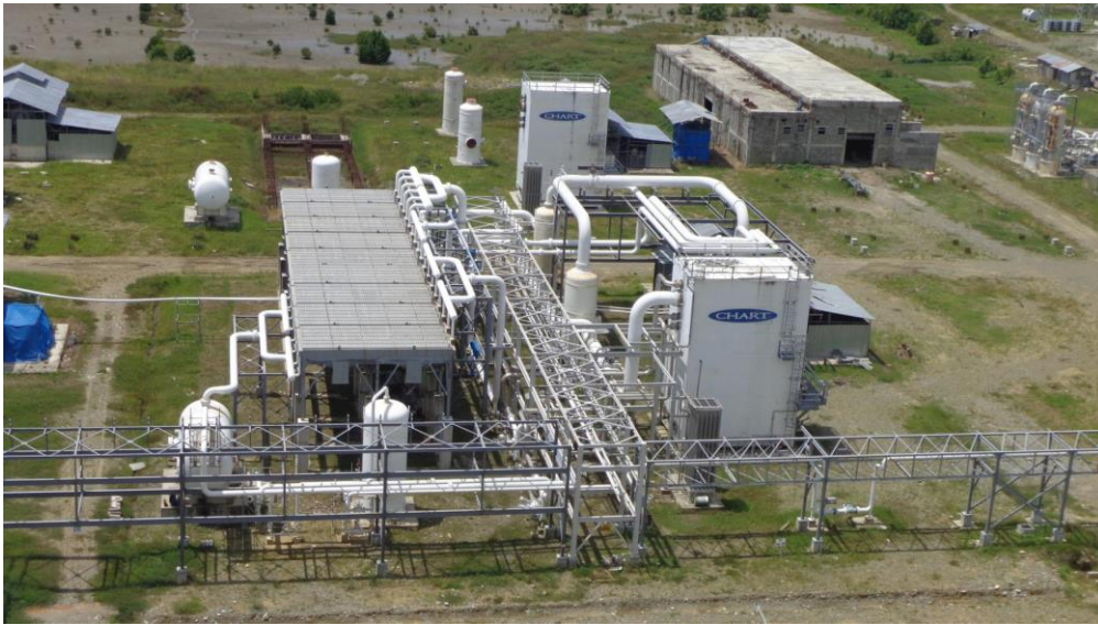
Main Processing Plant Area
