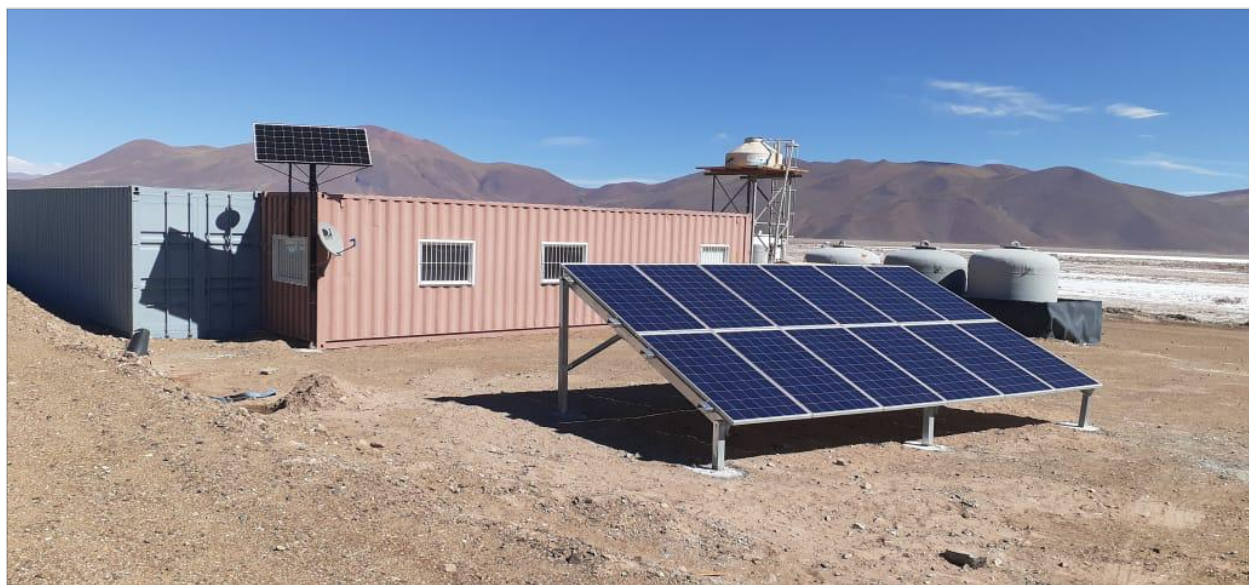
Figure 4. Rincon Lithium Project – Installed Solar Panels Providing Power on Site
