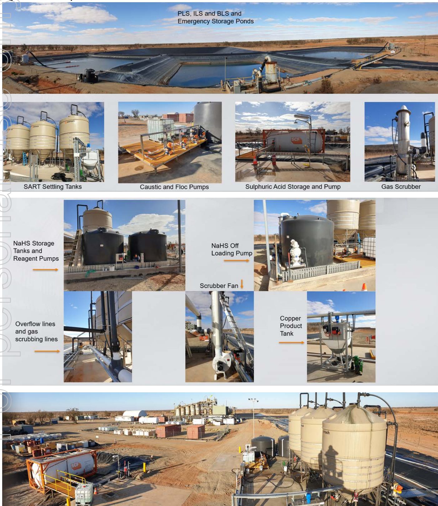
Figure 1: Process ponds and new SART Plant
