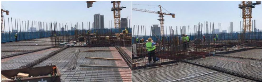
Installation Formwork and Rebar to Beam and Slab - PPCC T1 Zone 2 Level 12
