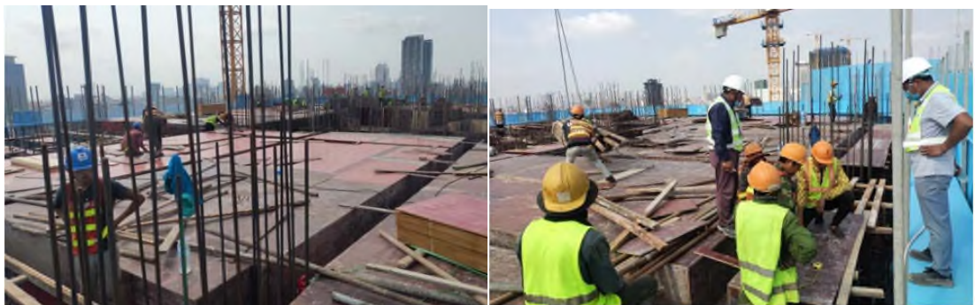
Installation Formwork and Rebar to Beam and Slab - PPCC T2 Zone 3 Level 12
