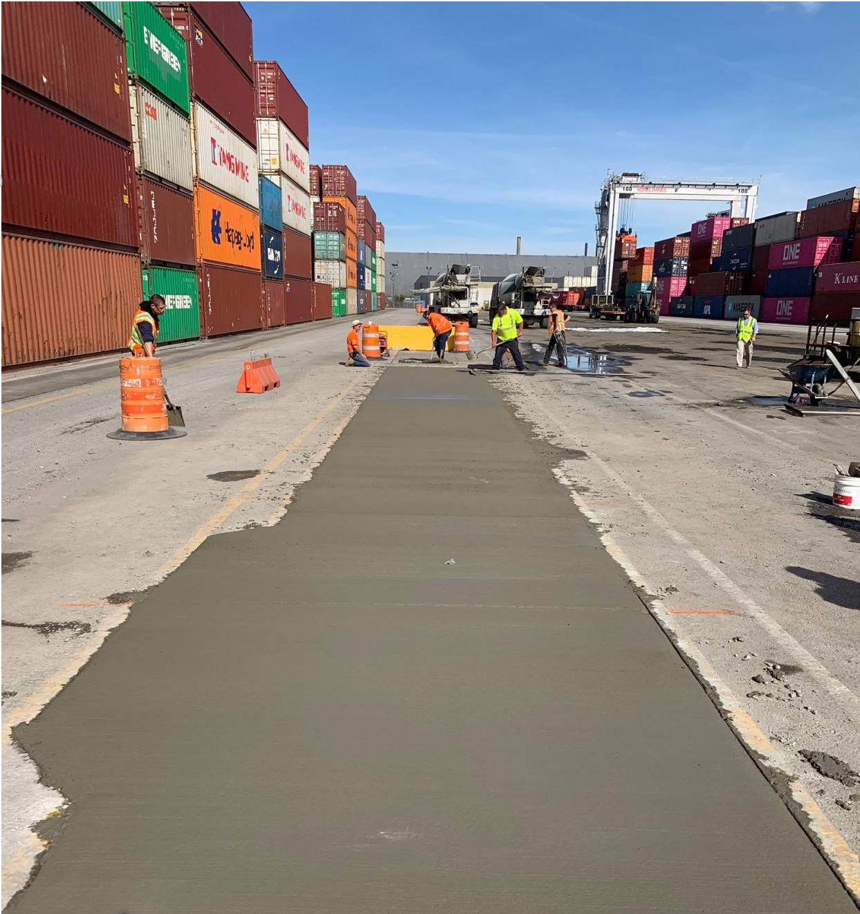
Figure 2. EdenCrete®- enriched concrete being poured at Garden City Terminal, Port of Savannah
