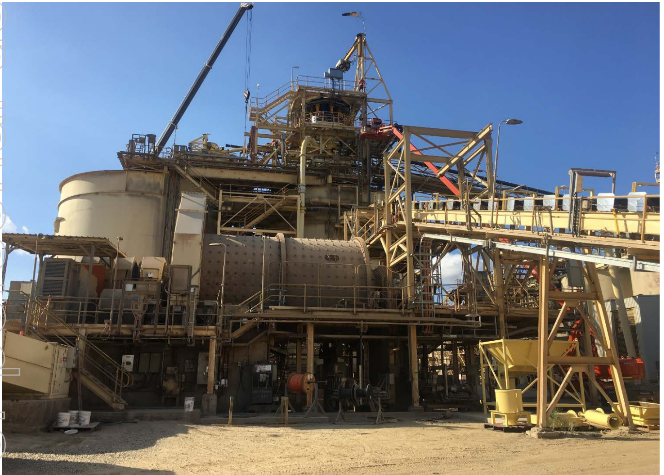
Figure 10: Nolans Processing Plant with third grinding mill (Mill #3)
