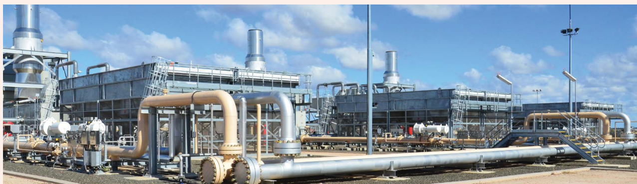
Wallumbilla Compressor Station in Queensland
