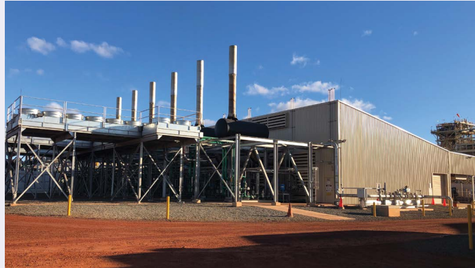
Gruyere Power Station connected to the Yamarna Gas Pipeline in Western Australia
