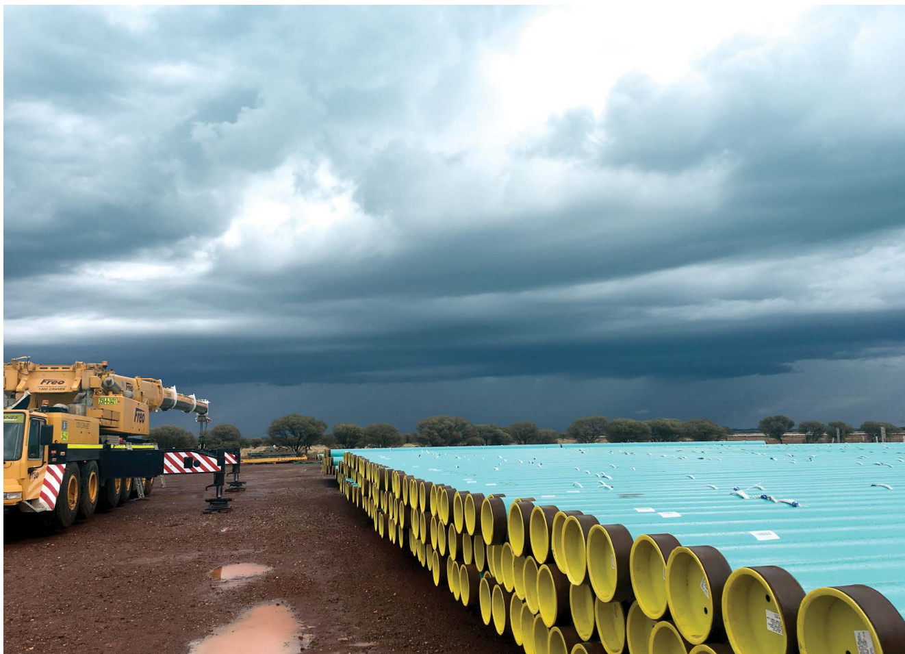
Pipe laydown for the Murrin Murrin Lateral looping project in Western Australia
