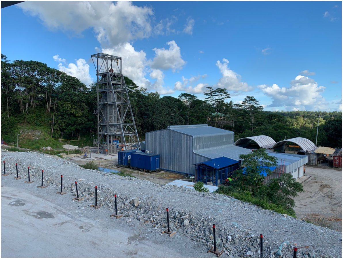
Figure 1: Completed E15 Service Shaft and surface infrastructure
