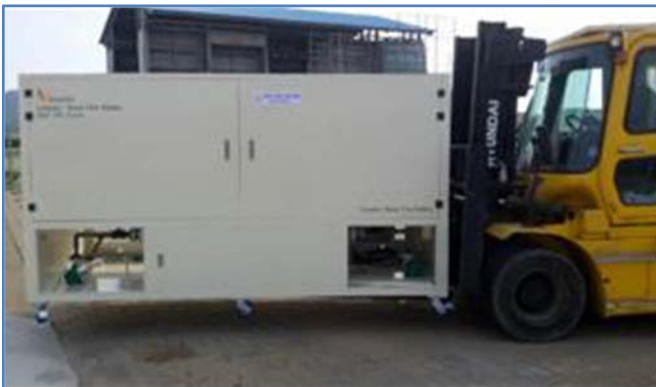
Fig 1: 50kW VRFB-ESS (2x25kW) deployed at solar test site
