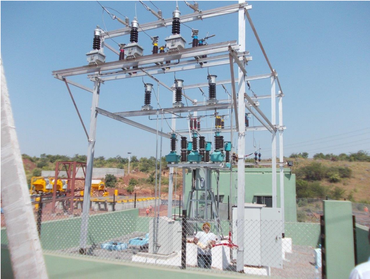
The moment of energisation
