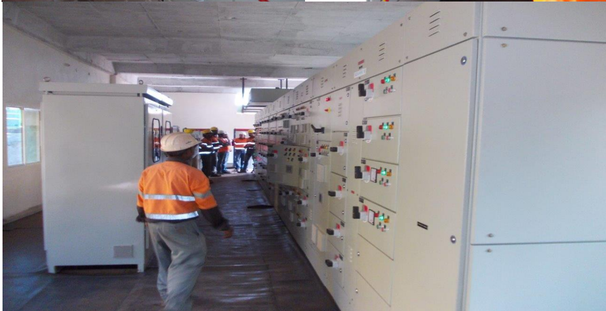
Powered Motor Control Centre (PMCC) Panel powered up
