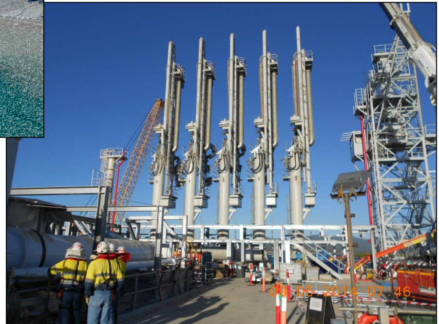
Loading Arms installed on Platform
