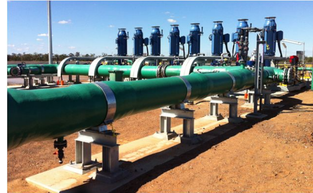
Condabri Central - Feed Pump Station
