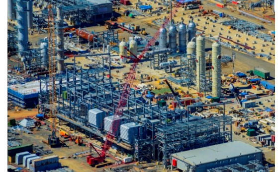
Overview of Train 1 Inside Battery Limits (ISBL)
