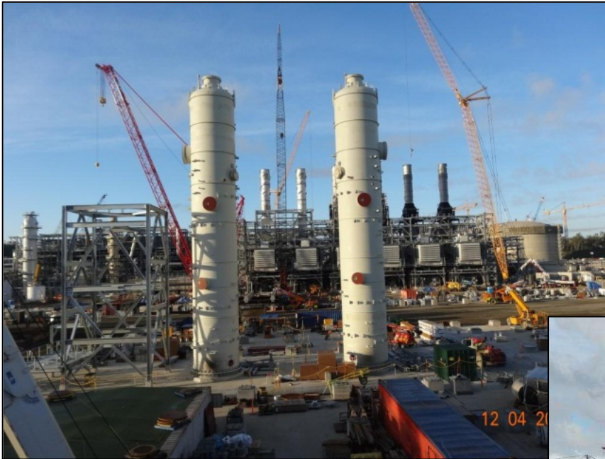
Propane Suction Drums Set
