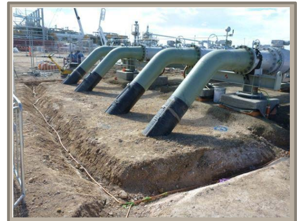
Inlet risers at gas processing facility
