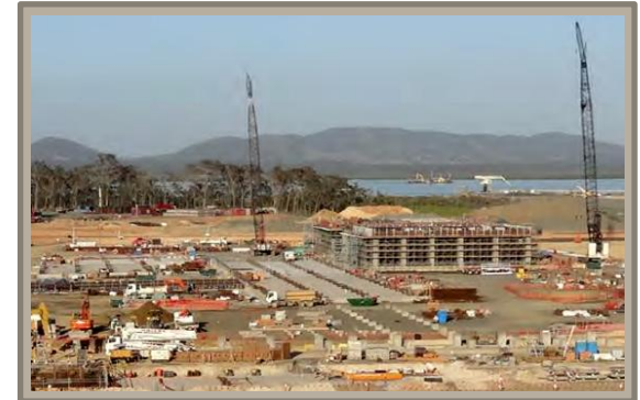
Overview of Train 1 Inside Battery Limits (ISBL)
