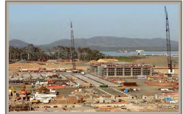
Overview of Train 1 Inside Battery Limits (ISBL)
