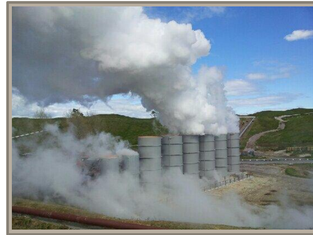
Steam Field 2 Dump Station (Te Mihi) being used for the first time
