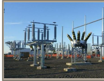
Condabri North Switchyard
