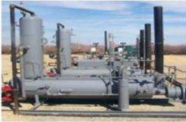
SGY 100% SELH Gas Production Facility
