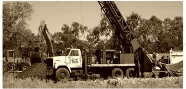
RC drill rig finishes one hole whilst next drill pad is prepared
